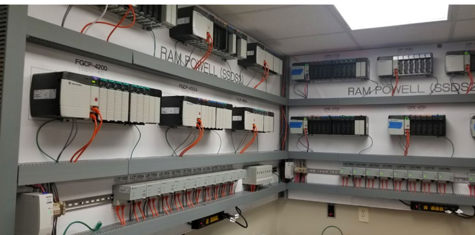
W-Industries' new hardware is staged prior to shipment to the asset for installation. (Source: W-Industries)
