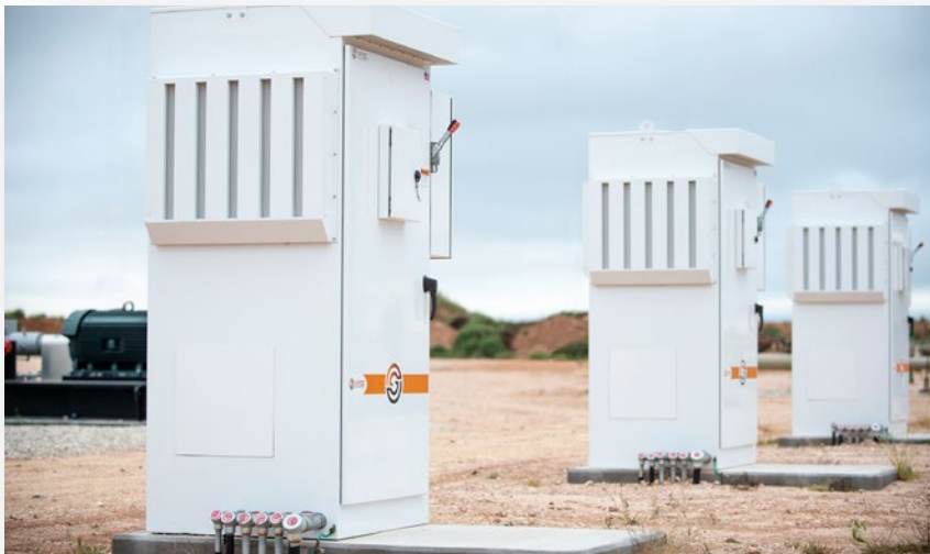
Three VFDs in a midstream water site control an array of horizontal pumps. (Source: SPOC Automation)
