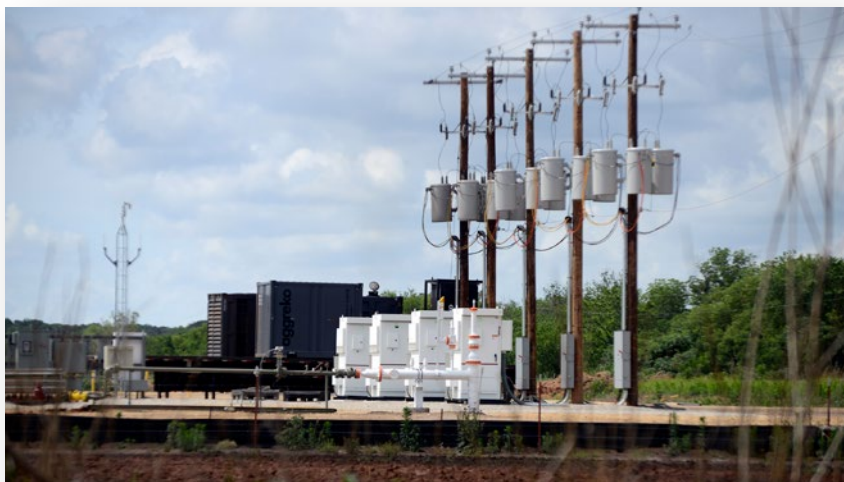
A bank of VFDs controls an electric submersible pumps site. (Source: SPOC Automation)
