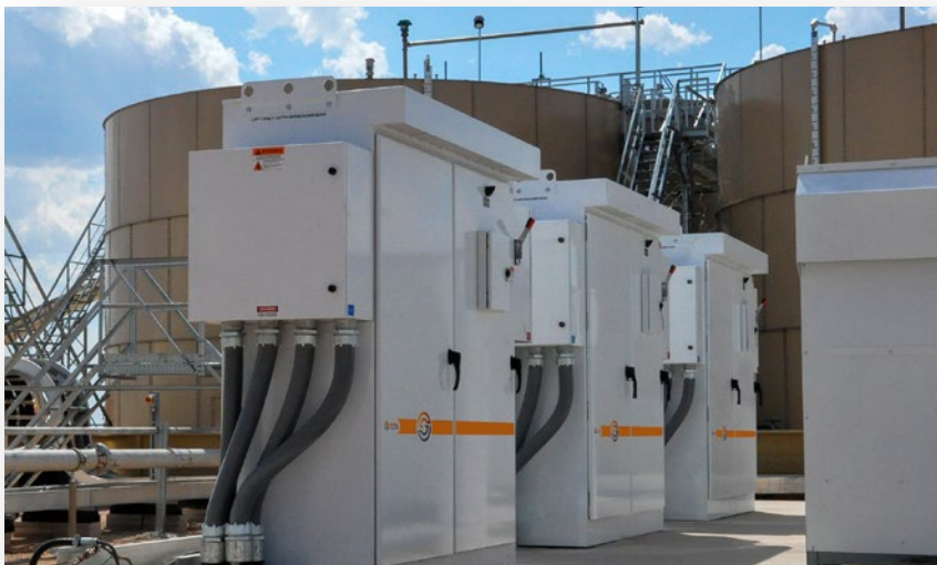
VFDs in a midstream water application operate outside of Midland, Texas. (Source: SPOC Automation)
