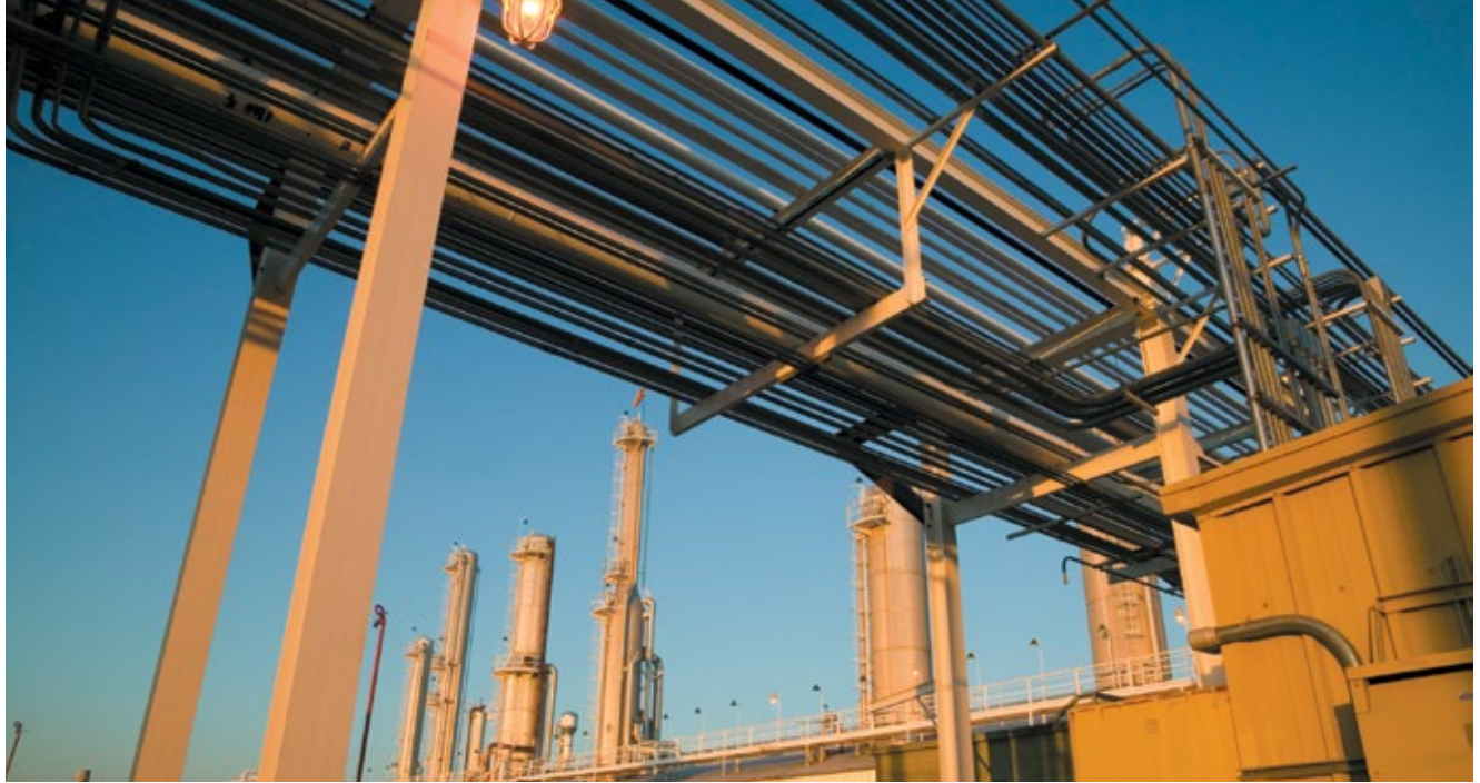
The Opal, Wyo., gas processing plant, part of Williams' Northwest Pipeline system, also serves as a major pipeline and storage hub for the Intermountain West. Source: The Williams Cos. Inc.
