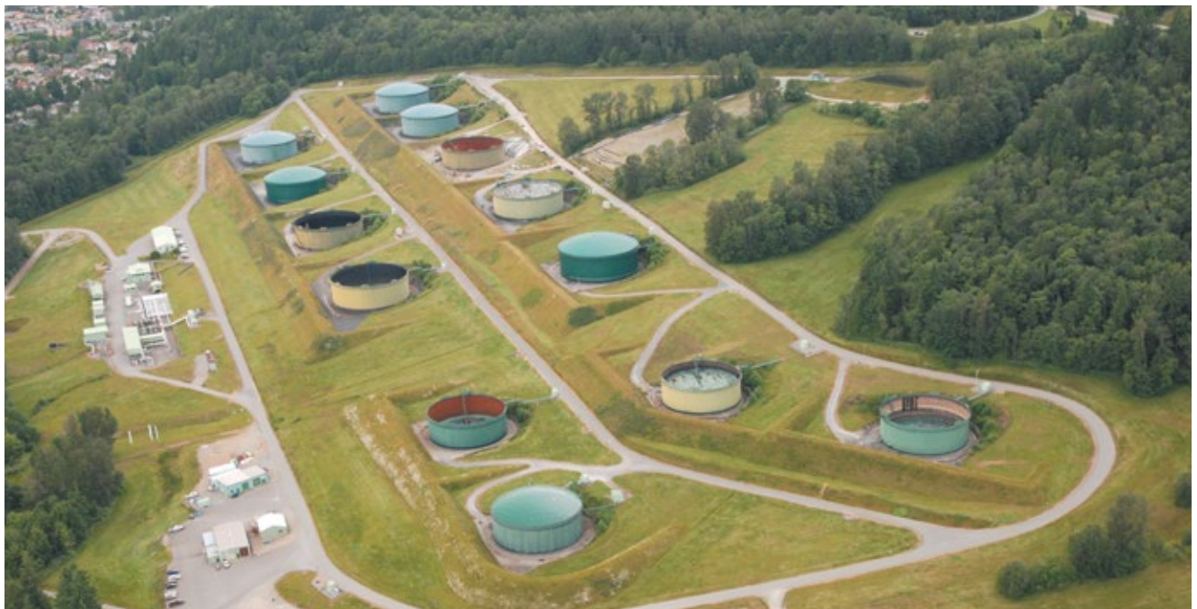
The Burnaby Terminal outside Vancouver has been in service since 1953. It is the end point of the only North American crude pipeline to reach the Pacific. Source: Kinder Morgan Canada
