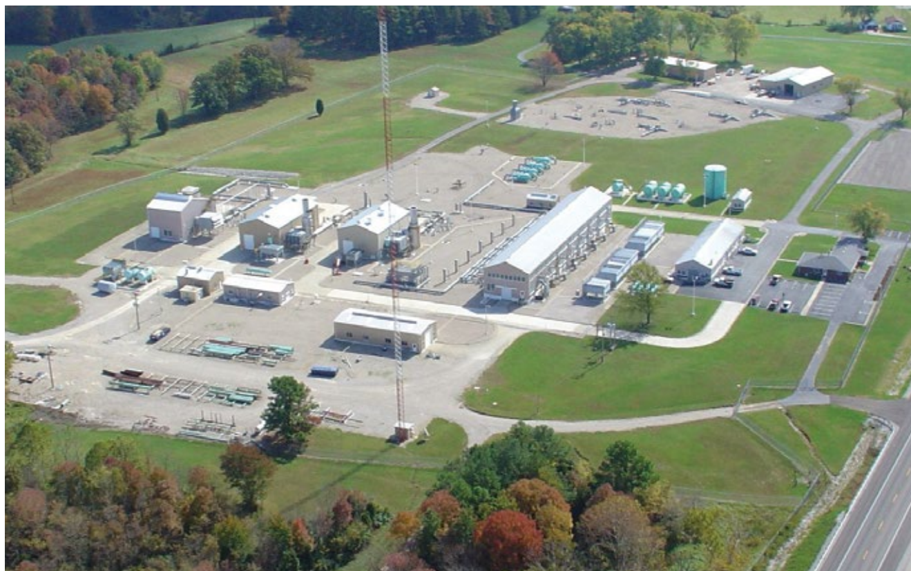
Boardwalk Pipeline's Hardinsburg, Ky., compressor station keeps gas flowing through its Texas Gas Transmission system.
