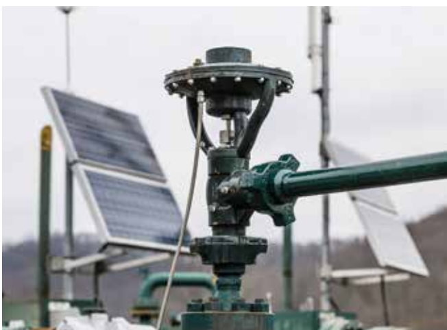
Nearly 9,000 pneumatic controllers were replaced or retrofitted with primarily electric actuators and air compressor installations on all EQT production locations and compressor stations.
