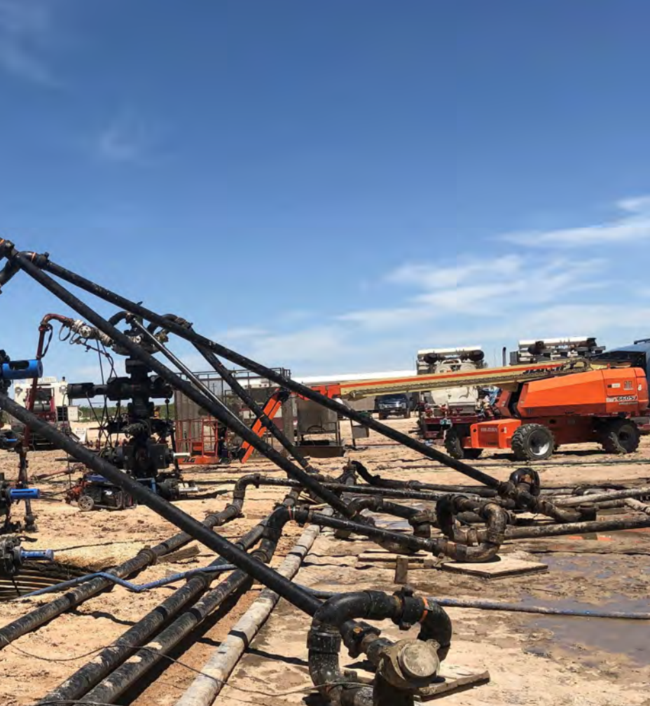
A workover rig drills out frac plugs on Hibernia Resources' six-well UL Boss Hogg pad in central Upton County, Texas. (Source: Hibernia Resources)
