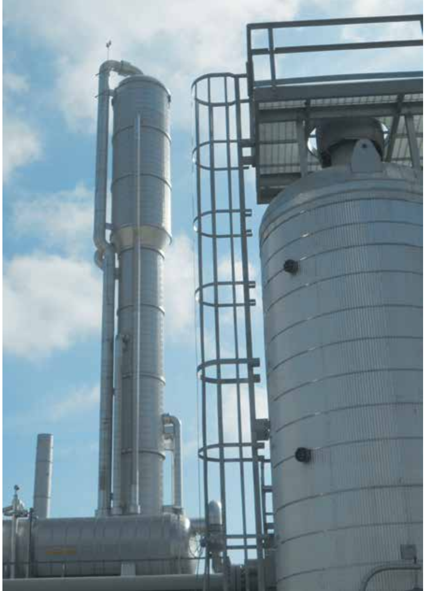
This Targa processing plant in Wise County, Texas, serves Barnett Shale producers. The firm has been a perennial top player in gas processing and NGL production. Source: Hart Energy
