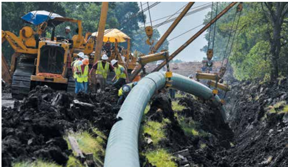
Workers lower 30-inch pipe in the ditch, part of Aspen Midstream's Giddings Field expansion in South Texas. Source Aspen Midstream LLC
