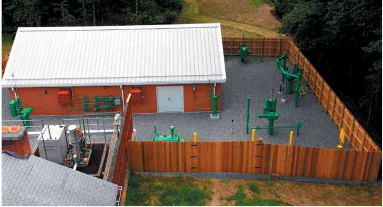
Midstream operators work to blend in with the wooded countryside typical of Appalachia. This station serves the Transco system's new Rivervale South to Market line that entered service earlier this year. Source: The Williams Cos. Inc.
