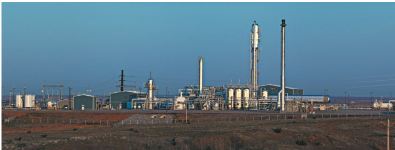
Enable's cryogenic McClure plant in Custer County, Okla., offers 200 million cubic feet per day of capacity to Anadarko Basin producers.
