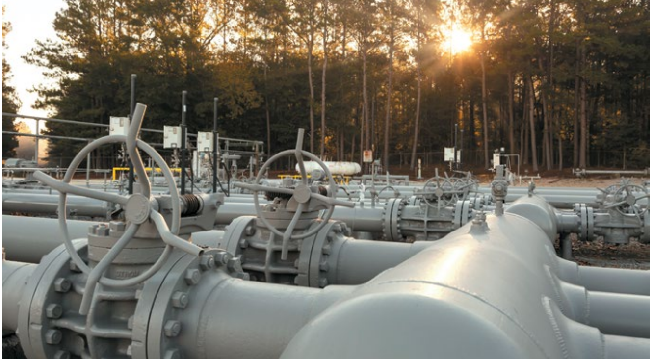
Enable Midstream Partners LP's Arkoma District serves producers in eastern Oklahoma and Arkansas. Its gas transmission network reaches from Oklahoma to Illinois and the Gulf Coast. All photos, Enable Midstream Partners LP
