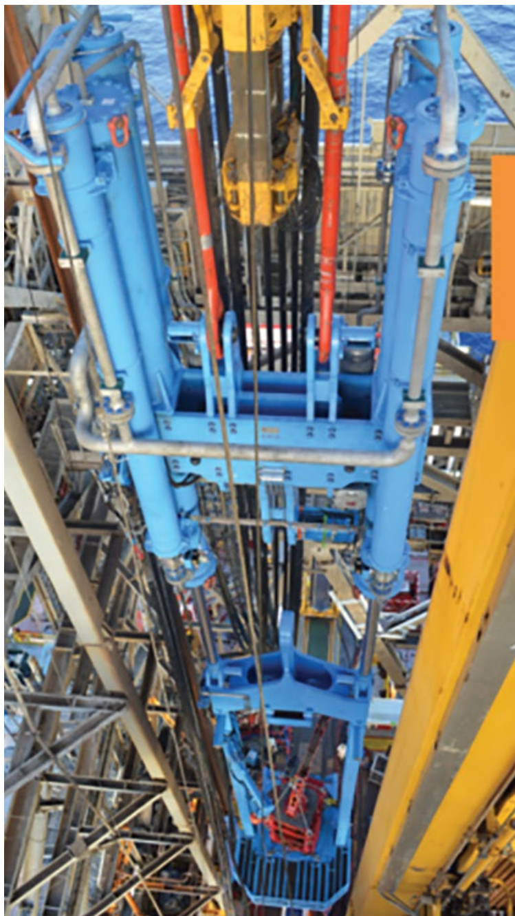
This soft rope traction winch has been in service offshore for more than 11 years. (Source: Logan Industries)
