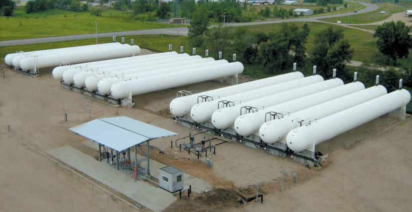
Fifteen 90,000-gallon propane storage tanks serve the truck rack in the foreground at a recently opened CHS Inc. rail terminal in Glenwood, Minn.
