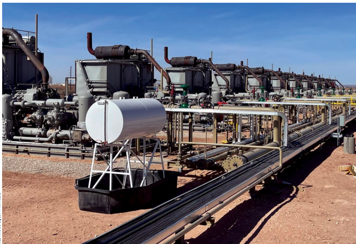
The Herradura compressor station is Crestwood's newest station, with capacity of more than 100 MMcf/d. It was commissioned in April.
