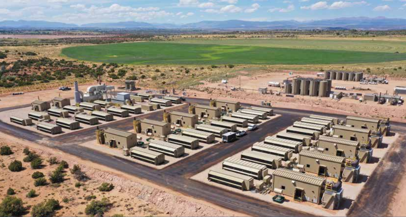
XCL Satoshi pad with Crusoe fully deployed. In the left portion of the image, there is a single large natural gas-powered turbine that provides about 50% of the site's power. On the right side of the picture are 10 natural gas engine generators that supply the remaining half of the site's power. Each of these natural gas engine-driven generators can support two bitcoin mining containers, with each container housing approximately 220 individual bitcoin miners. The pad covers an area of approximately 10 acres and consumes around 5.5 MMcf/d of natural gas.
