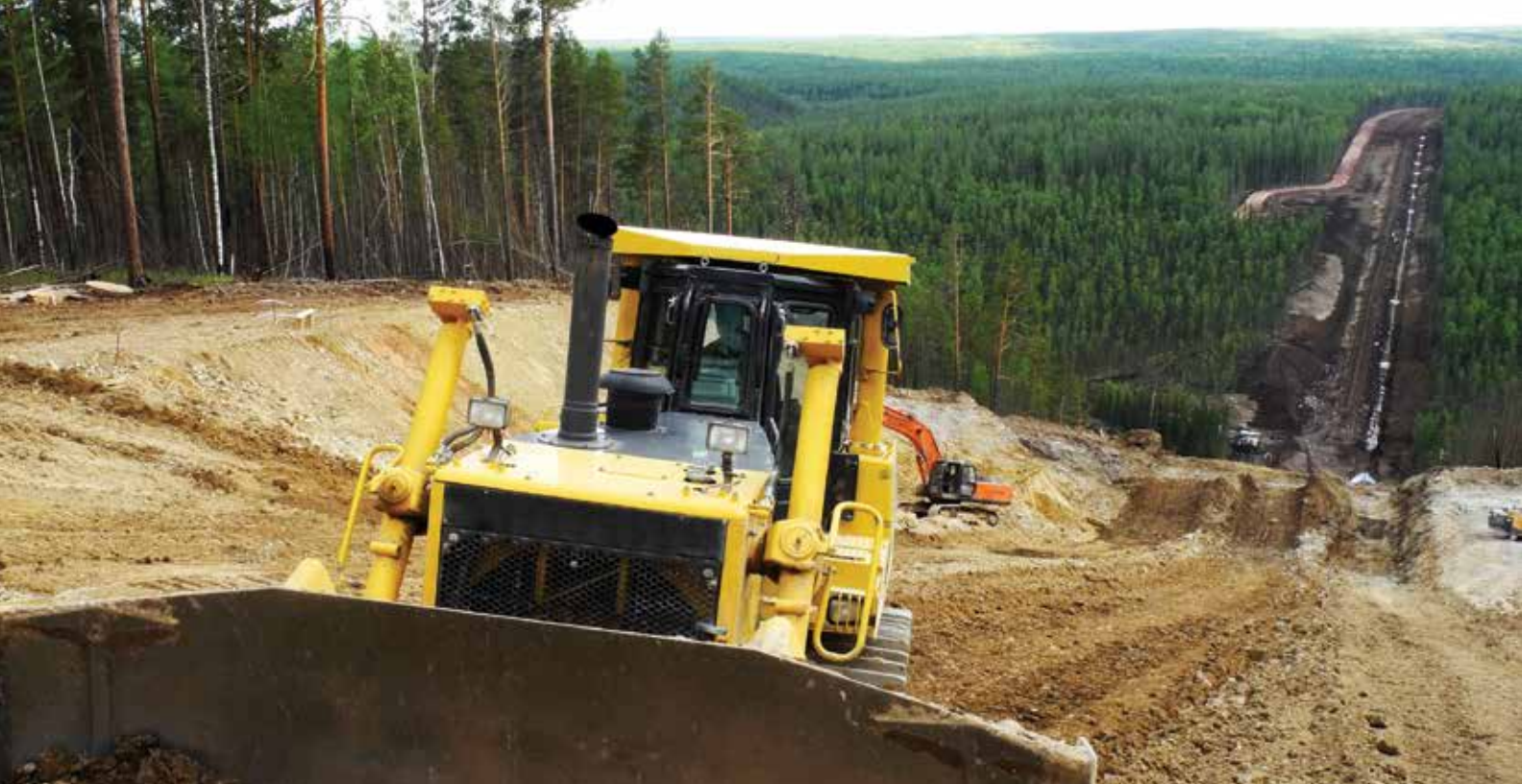
Construction of the Mountain Valley Pipeline, an interstate natural gas pipeline, near Cowen, W.Va.
