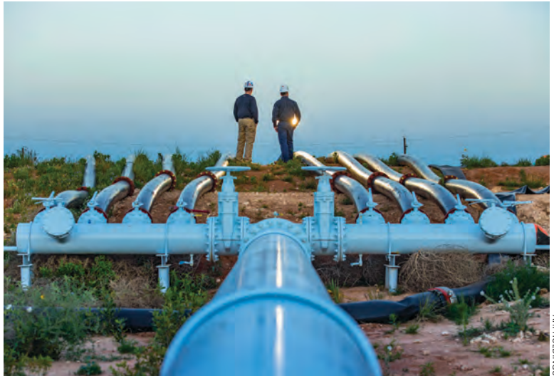
XRI Holdings operates more than 350 miles of permanent pipelines throughout the Permian Basin.
