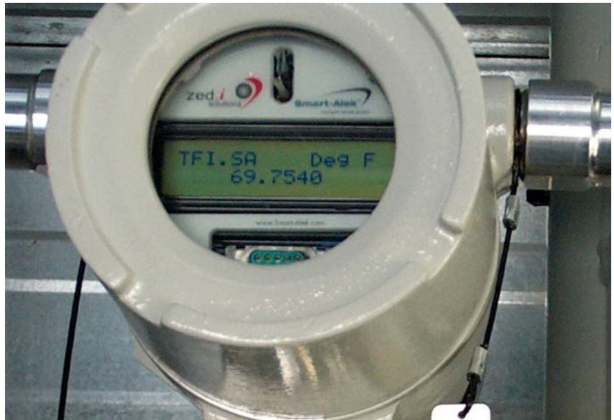
The local display on the Smart-Alek unit allows operators to view gas flow parameters in real time.
