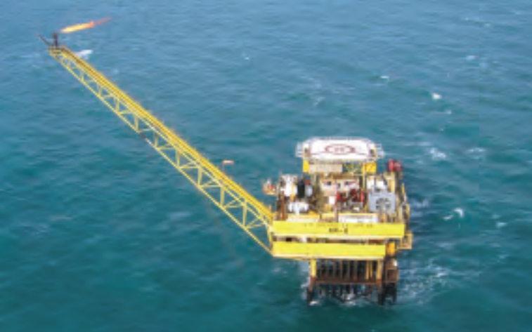
Mechanical mounting and instrumentation on an offshore platform in the Magellan Strait. (Photo courtesy EDVSA)
