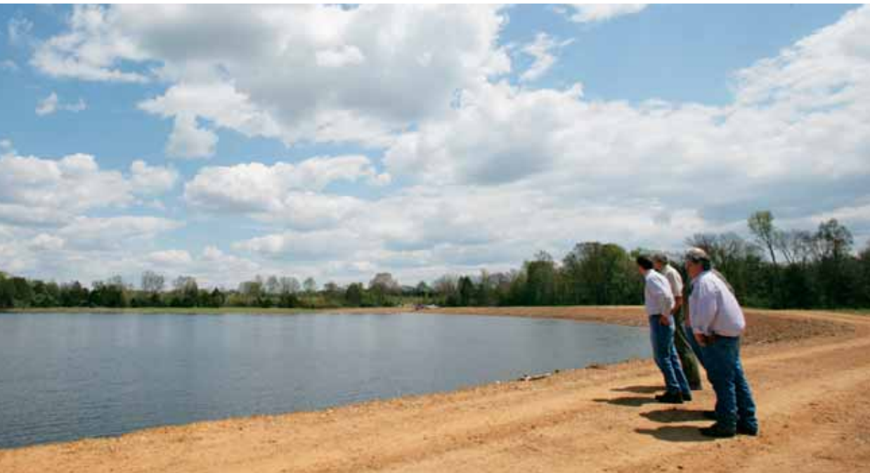
One of 28 ponds that Seeco has constructed in the Fayetteville play is a source for frac water.
