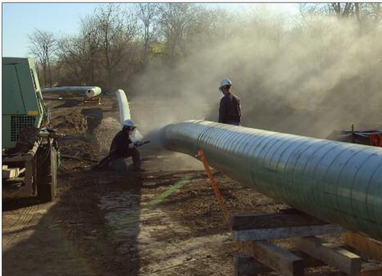
Crosstex Energy has added to the available Barnett Shale takeaway capacity with the completion of its North Texas pipeline project. Photo courtesy of Crosstex Energy
