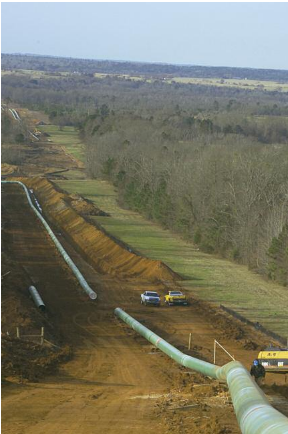
Enbridge Energy Partners completed work a few years ago on its US $530 million East Texas expansion project, which involved 252 miles of 36- and 24-in. pipe and the construction of a new gas-processing plant in Franklin County. Photo courtesy of Enbridge Energy Partners
