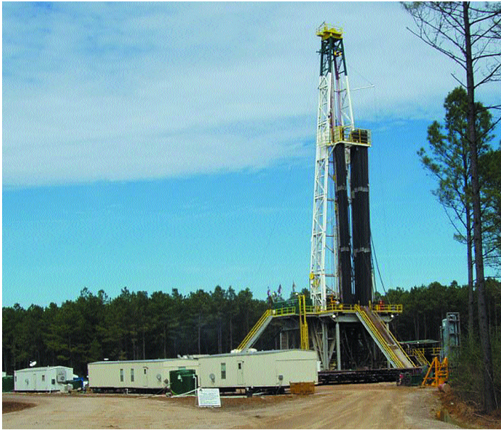
In February, Grey Wolf Drilling Inc. Rig No. 91 was drilling the 22,000-foot Anadarko Petroleum Co. Black Stone Minerals A-249 No. 1, a Deep Woodbine wildcat in Polk County, Texas.
