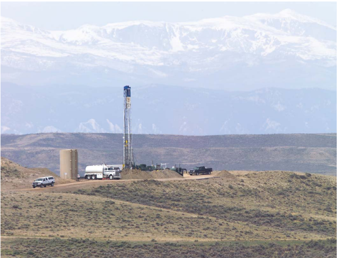
One of Devon Energy’s CBM drilling sites targeting the Big George formation in the Powder River Basin near Gillette, Wyo. (Photo courtesy of Devon Energy)
