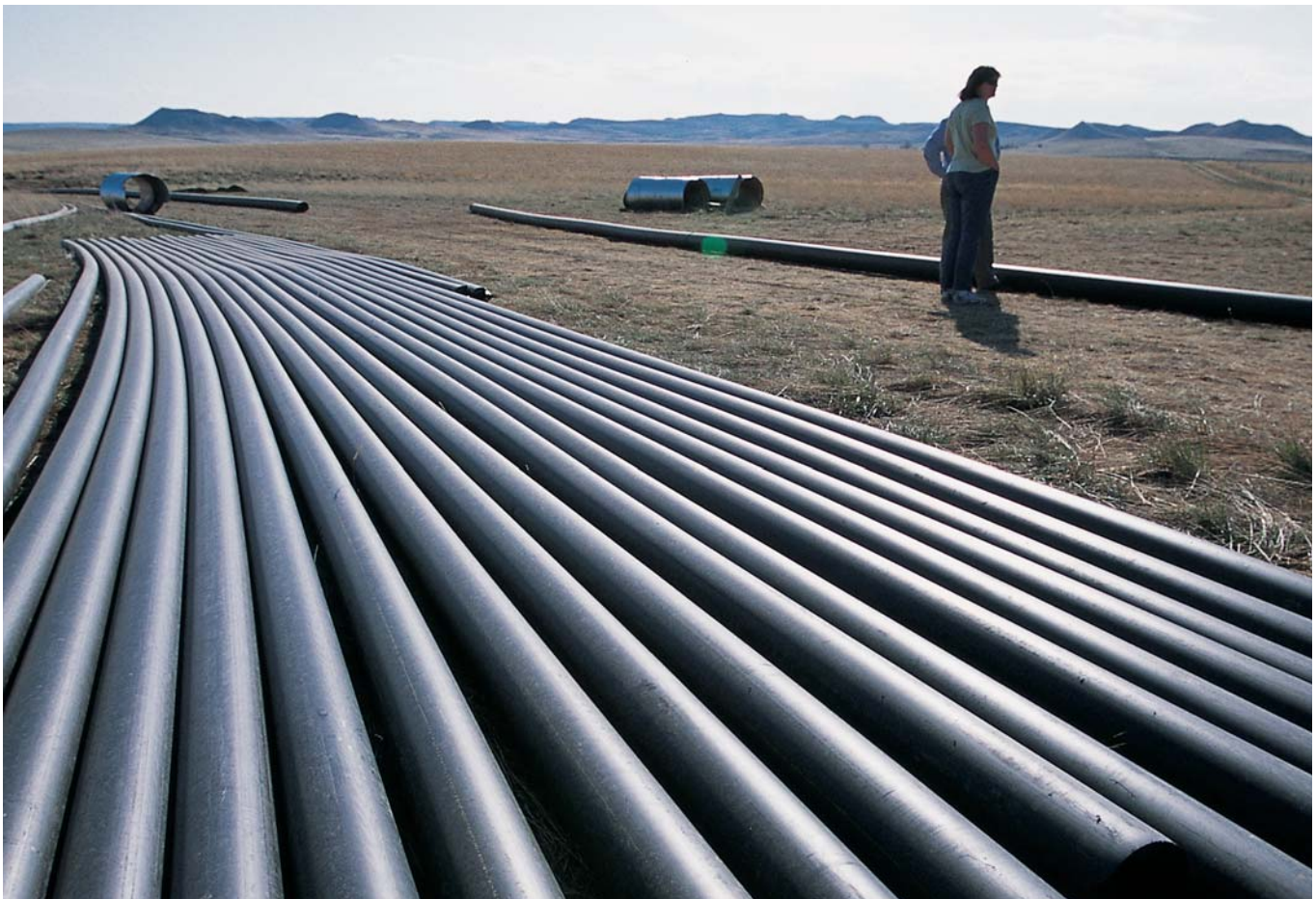
A stockpile of pipe awaits burial near a compressor station in Wyoming. The pipe will transport coalbed methane to a larger line. (Photo by Lowell Georgia)
