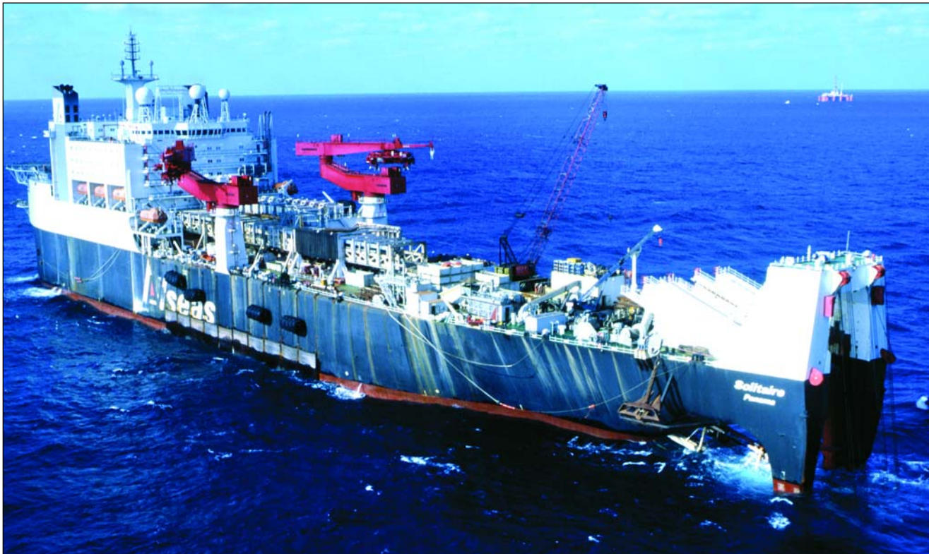
Industry proposes 1,600 miles of new gas pipeline alone. (Photo courtesy El Paso Energy Partners.)
