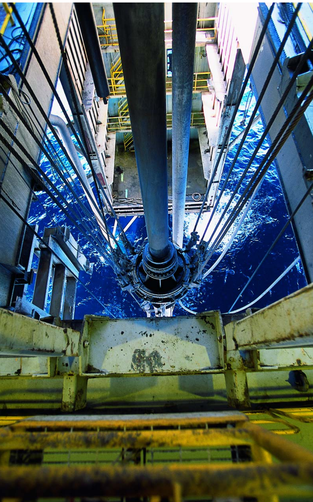
To be produced from a spar, the Devils Tower project has reserves of 75- to 100 million BOE. (Photo by Lowell Georgia.)
