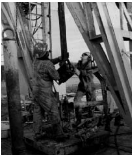
Roughnecks prepare to put a section of pipe down a new well underway in the 90-year-old Lawrence Field in Illinois.
