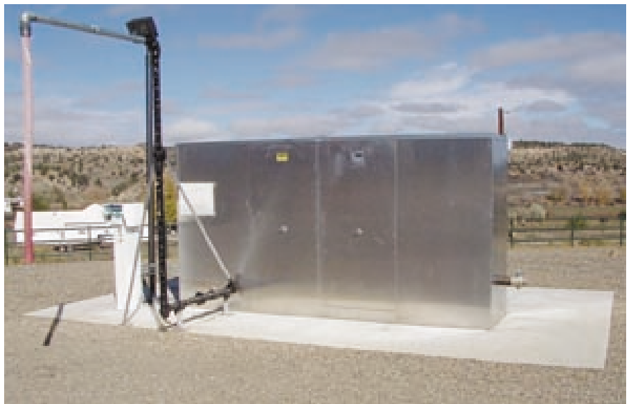
Evergreen Resources is converting CBM-well water into potable water and providing it via a new water facility in the Purgatoire River Valley.
