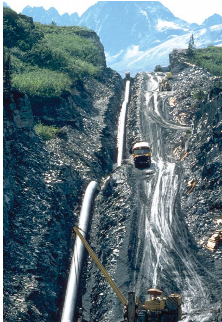
Pipe is shown below ground in this Alaska trench prior to burial.
