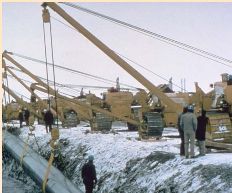
This crossing at the Tonsina River in the spring of 1975 was the first installation of pipe for the Trans-Alaska pipeline. The pipe was weighted with concrete anchors for burial below the river bed.
