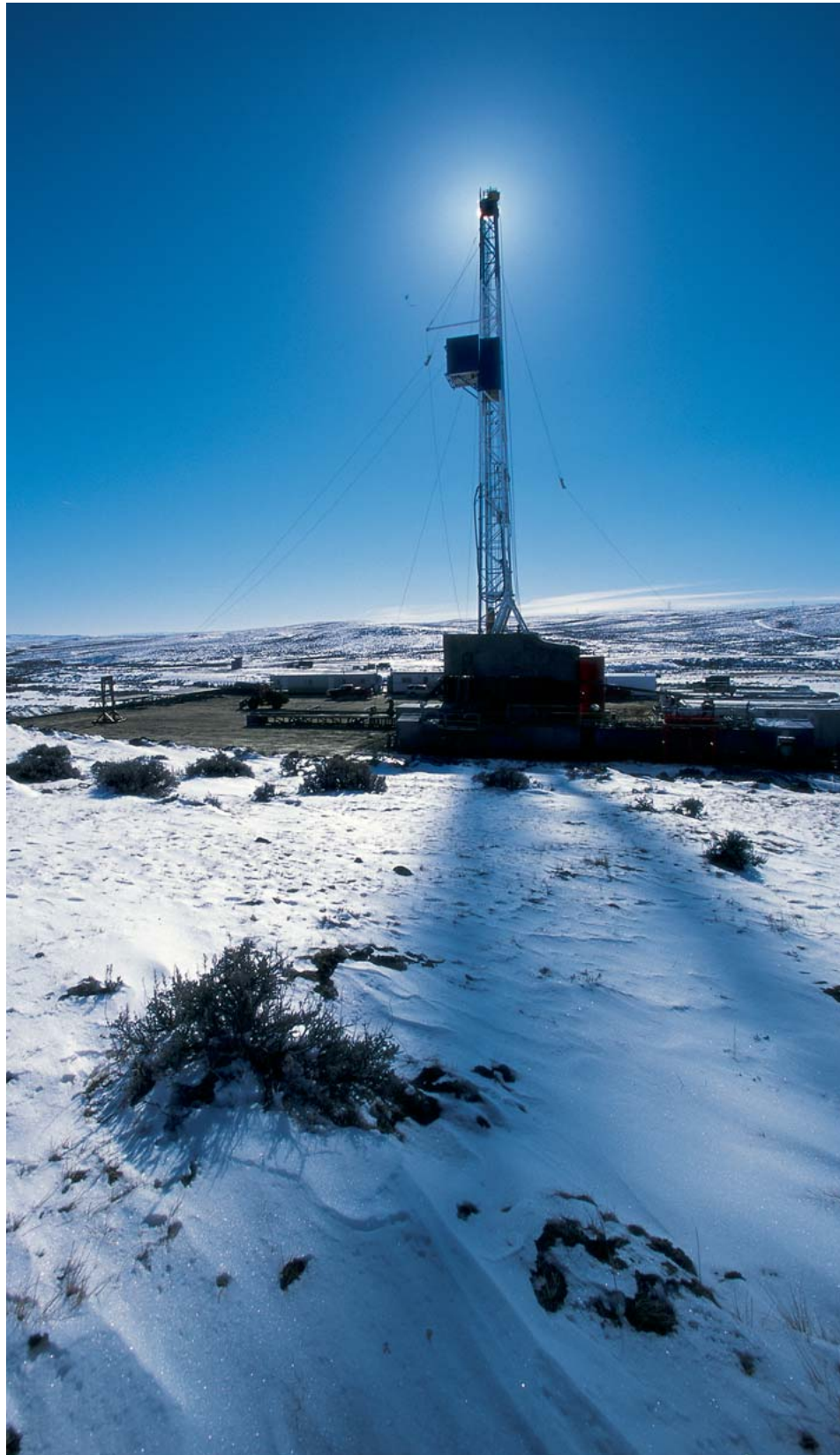
SST Energy Corp Rig #17 of Casper drills another gas well in the Coopers Reservoir, Natrona County, Wyoming.
