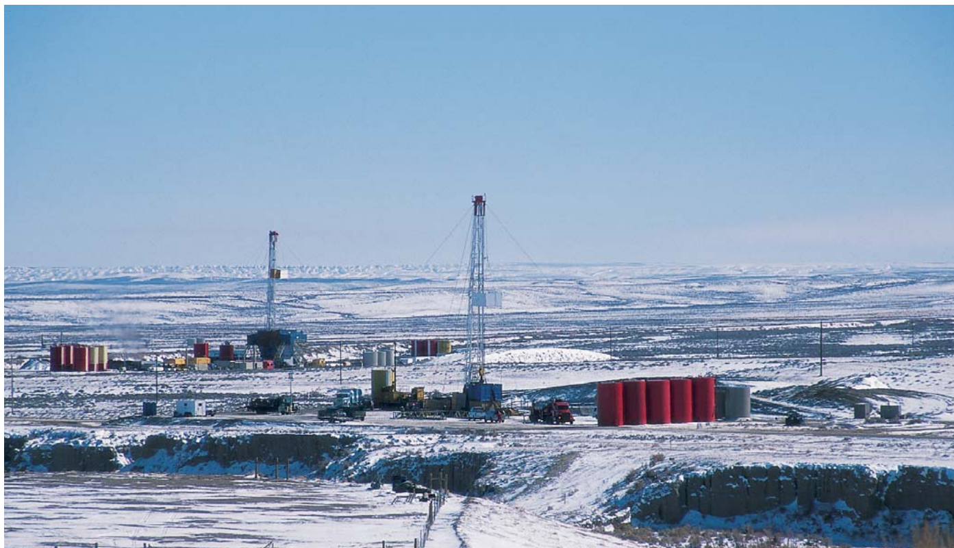
Two rigs complete natural gas wells for Bill Barrett Corp. in Wyoming's Cave Gulch field.
