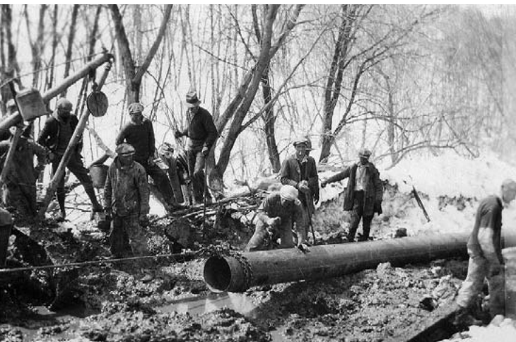
Pipeline construction crews faced the third coldest winter up to that time and snowfalls 50% greater than normal to lay a pipeline to Utah. (Photo courtesy of Questar Corp.)
