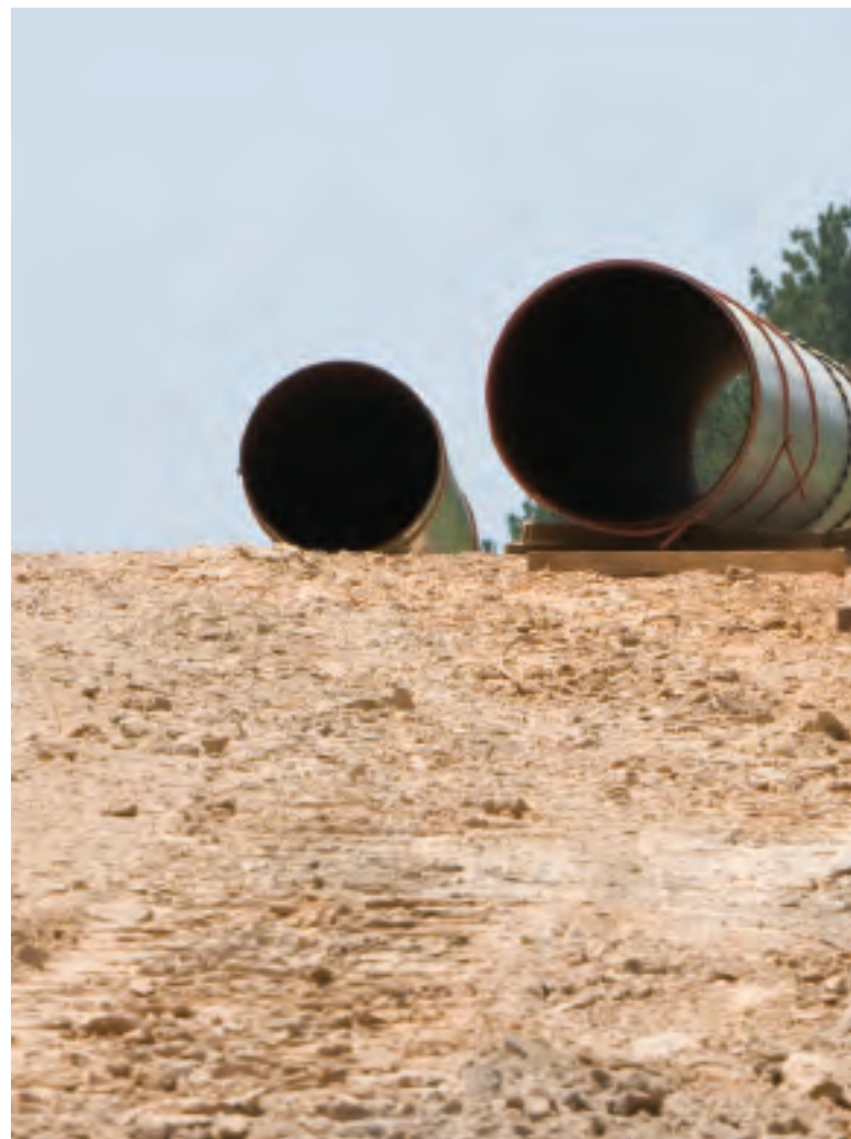
Pipes are set up and ready to go during construction of Regency Energy's Haynesville Expansion project.
