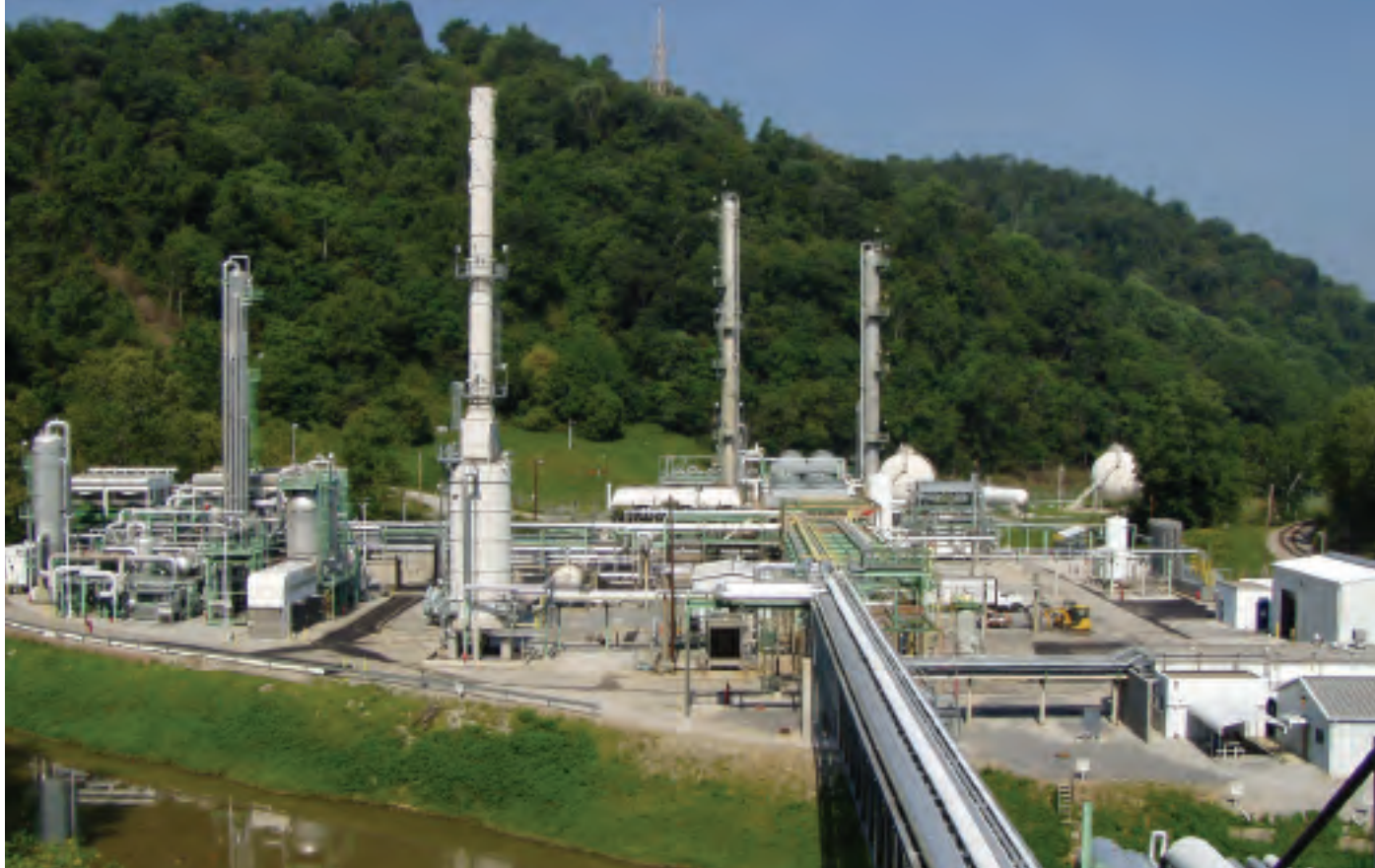
Dominion Transmission Inc.'s Hastings fractionation facility in Pine Grove, West Virginia, separates rich Marcellus gas liquids into propane, butane, ethane, natural gasoline and other liquids that are shipped to markets by pipeline, train, barge or truck.
