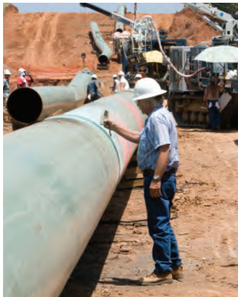
A coating inspector checks the millage on a pipe section of Regency Energy's Haynesville Expansion project.
