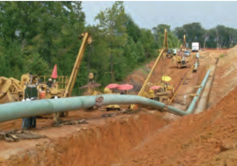
Crane operators lower pipes into a trench during construction of Regency Energy's Haynesville Expansion project.
