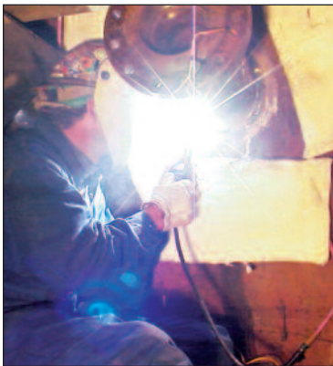
Installation of new nozzle (alloy material) on an existing refinery vessel by JV Industries Cos.
