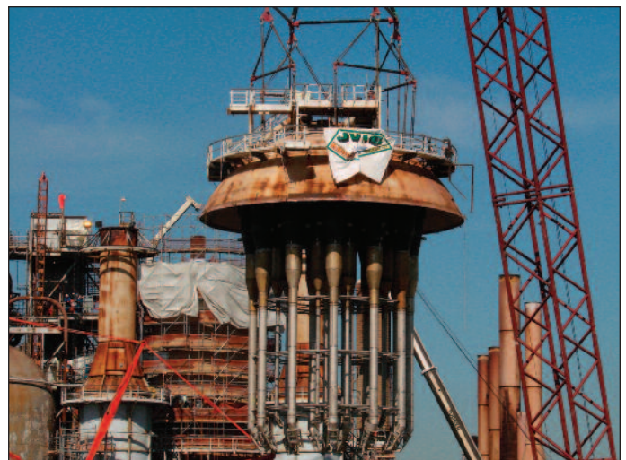
Refinery FCCU reactor vessel with new cyclones installed. Heavy-lift (200-plus tons) and cyclone change out by JV Industries Cos.
