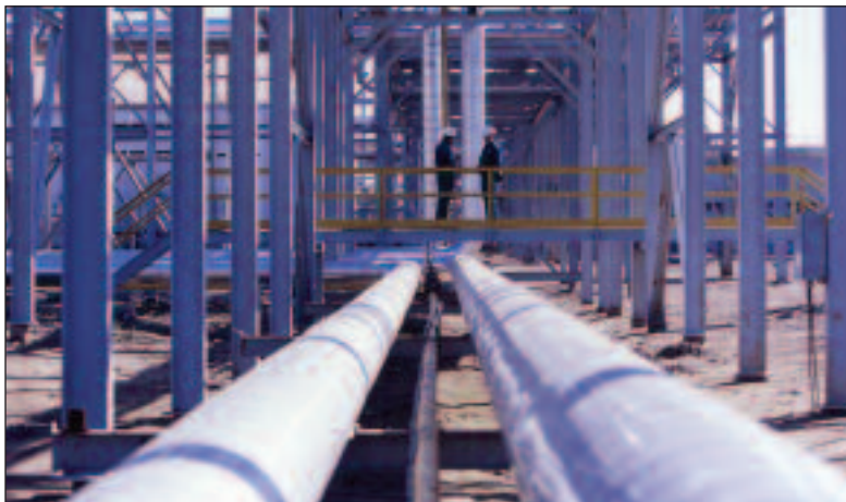
Canadian Natural's Primrose facility, Alberta, Canada.
