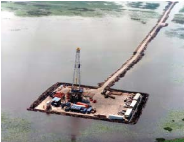
Newpark built the above temporary road and drilling location in the wetlands in Vermilion Parish, Louisiana. The company also supplies drilling fluids and environmental services (waste disposal).
