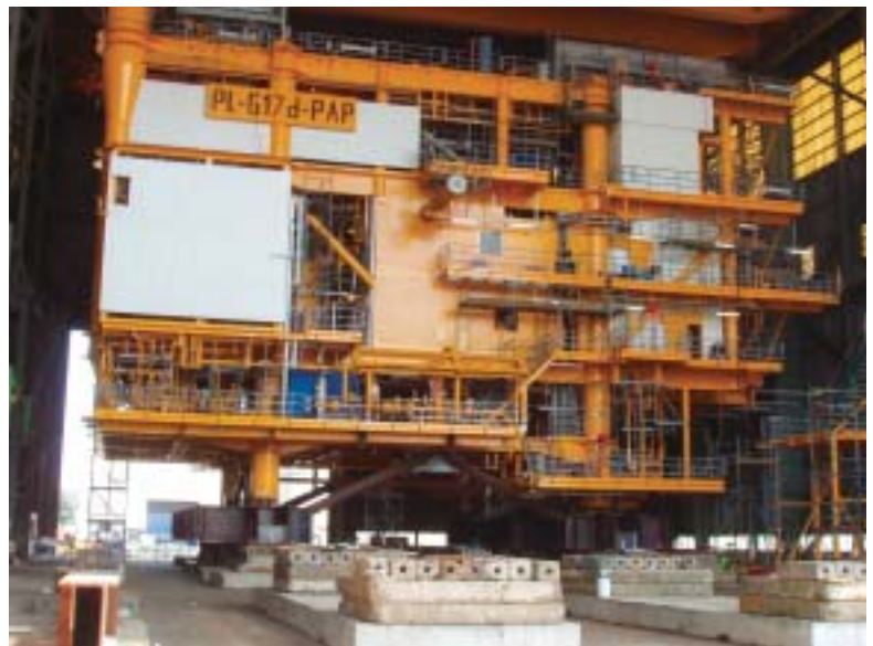
Production from the successful ATP Dutch sector North Sea L-06d natural gas well will tie into this G-17 processing platform currently under construction.
