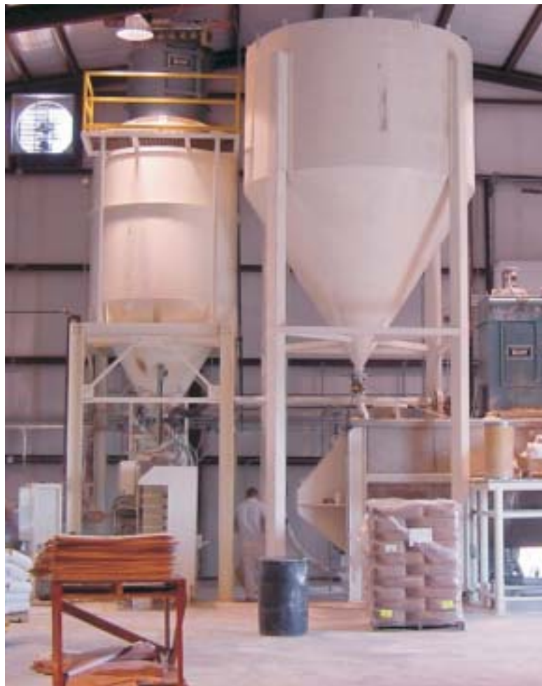
Flotek's Chemical division's dry blending facility in Marlow, Oklahoma.
