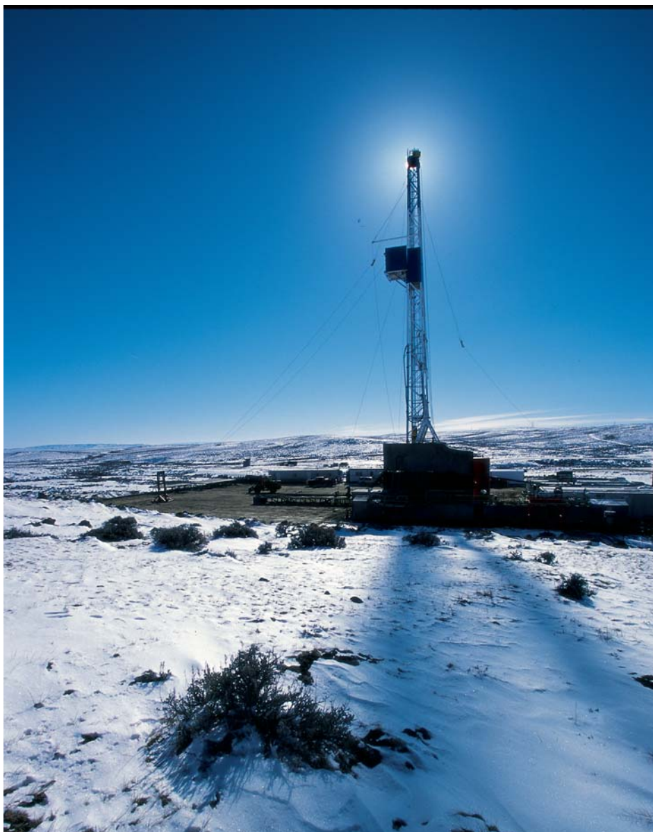
SST Energy Corp. Rig No. 17 of Casper drills another gas well for Bill Barrett Corp. in the Coopers Reservoir, Natrona County, Wyoming.
