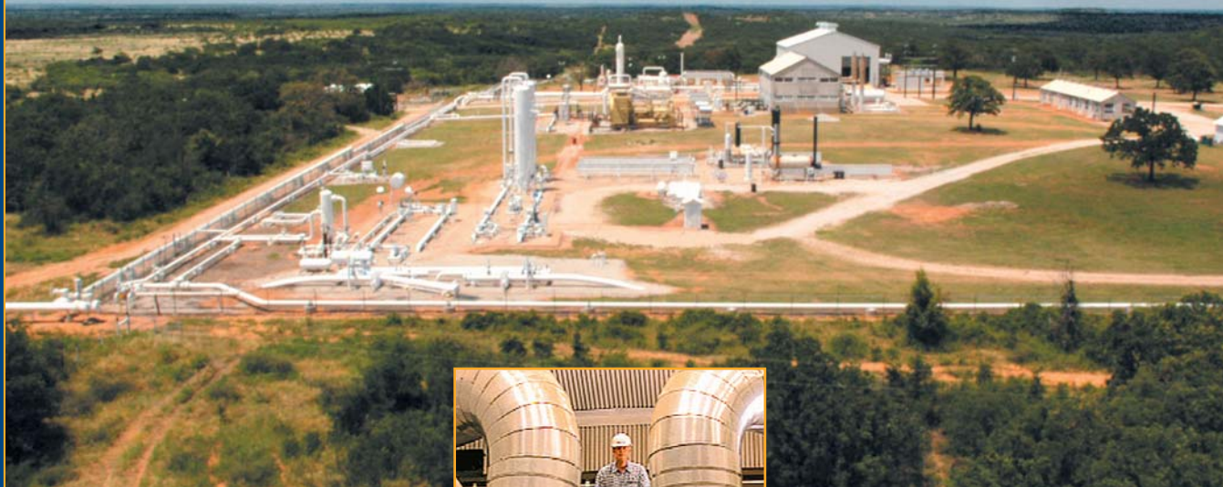
Hill-Lake Gas Storage Facility
