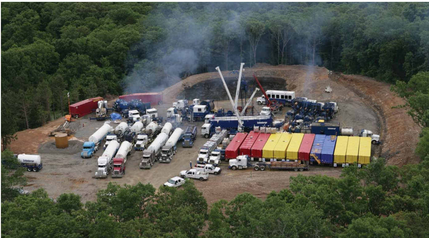
Schlumberger crews are performing one of four stages in a nitrogen-foam fracture stimulation on Southwestern Energy's McNew No. 3-2H horizontal well in Conway County. (Photo by Lowell Georgia)
