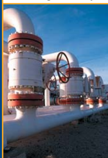
Worsham-Steed Gas Storage Facility
