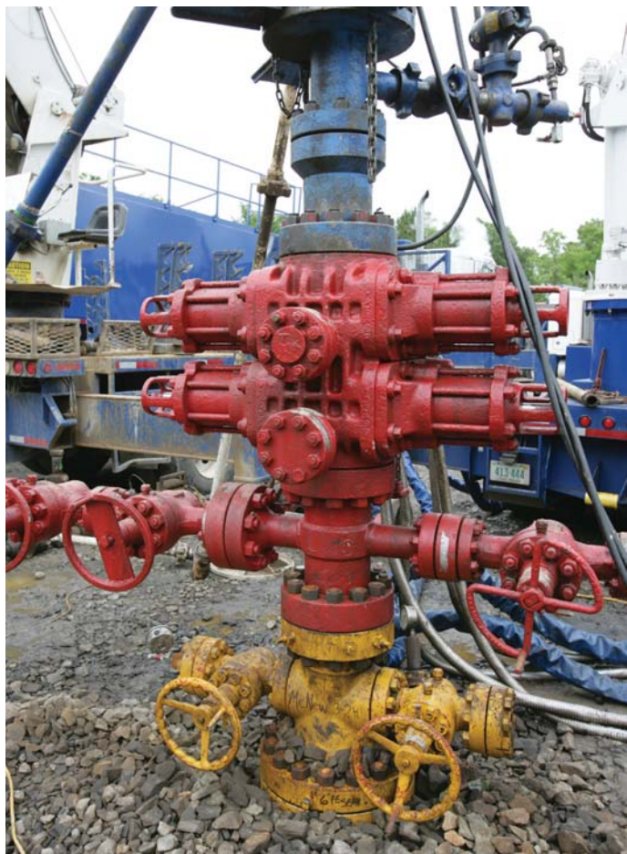
Southwestern Energy's McNew No. 32-H is rigged for a nitrogen-foam fracture treatment. The well, in proposed Gravel Hill Field, has a 2,310-foot lateral. (Photo by Lowell Georgia)
