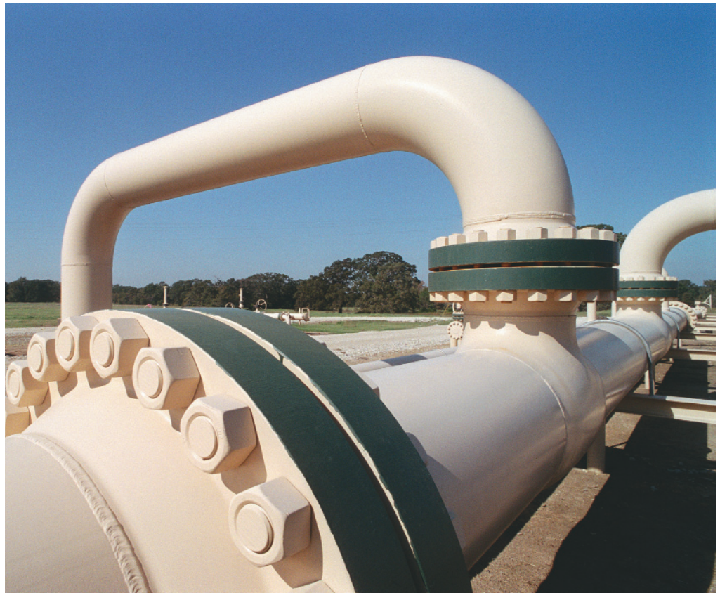
Compressor header for gas-gathering in the Freestone Trend. (Photo courtesy of XTO Energy Inc.)
