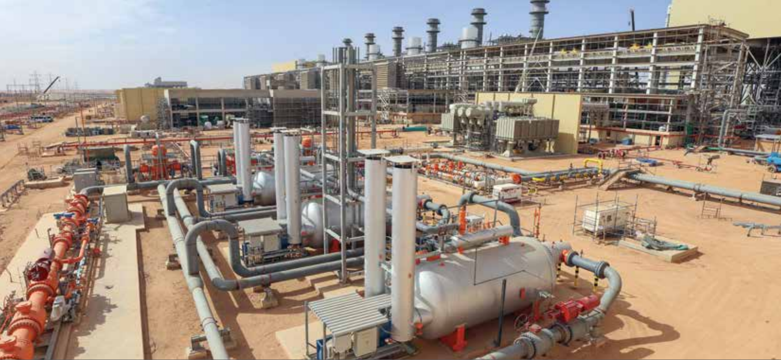
Construction of a modern combined-cycle gas turbine power plant. New construction of gas-fired power plants will be beholden to the new EPA regulations.
