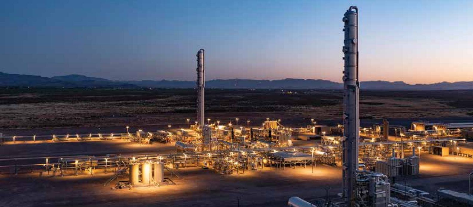
Kinetik midstream plant operating in the Texas Delaware Basin. Kinetik acquired Durango in early May, one of three Permian Basin deals this summer where a large public company bought out a smaller private with primarily natural gas gathering and processing facilities.
