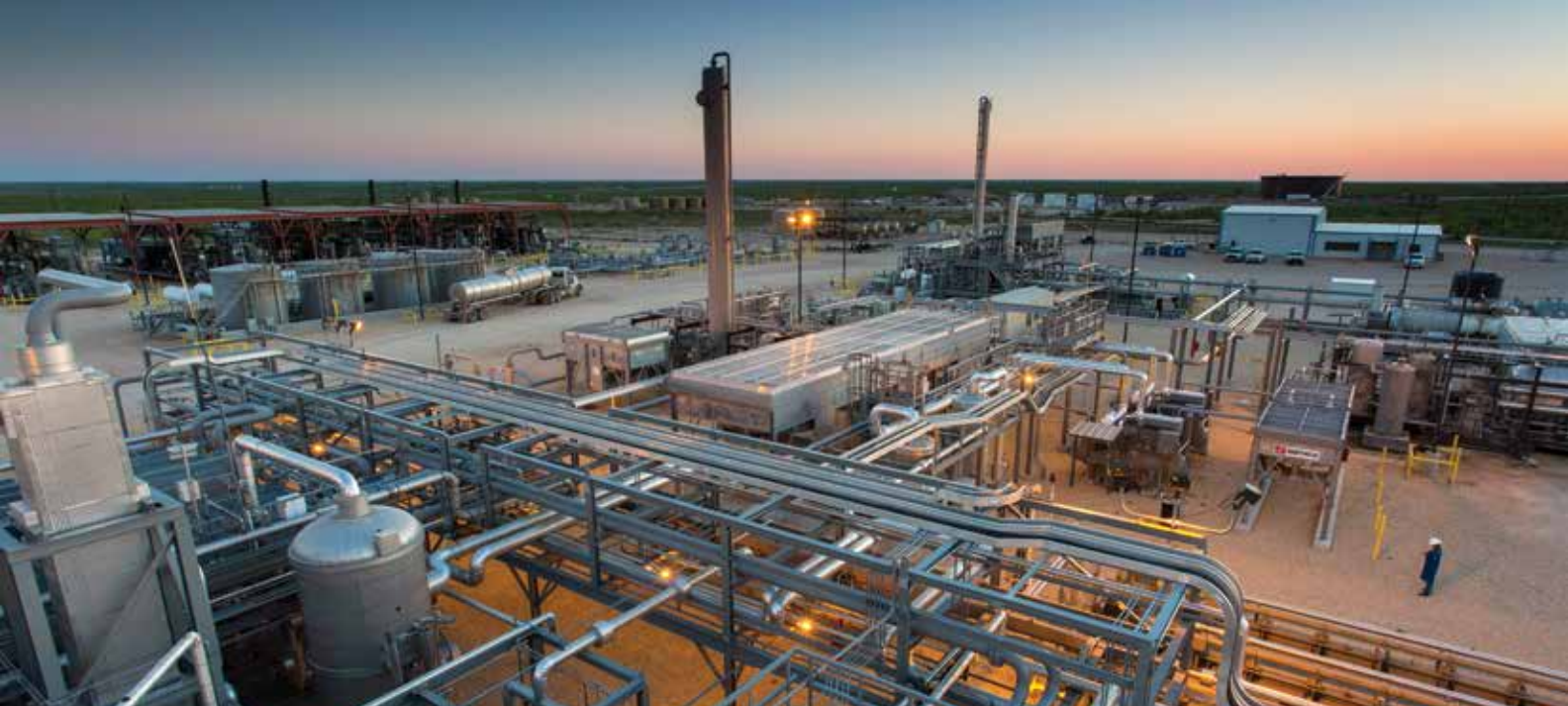
EnLink Midstream's Deadwood natural gas processing plant in Glasscock County, Texas.
