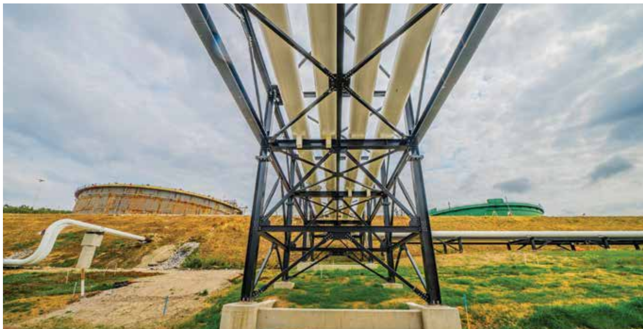
The end of the Trans Mountain Pipeline System, Burnaby Terminal, located just outside of Vancouver, Canada.
