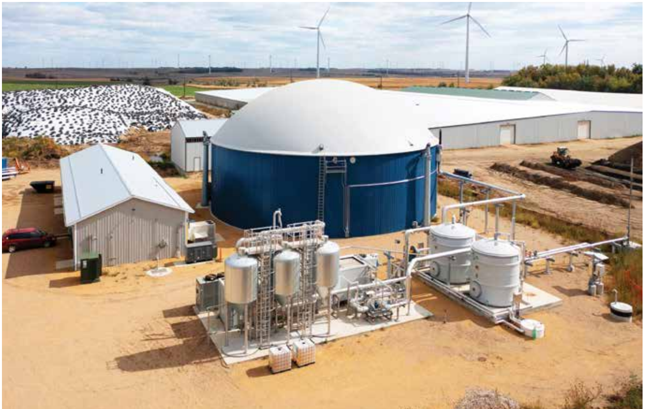
Clean Energy's RNG production facility at Ash Grove Dairy, Lake Benton, Minn.
