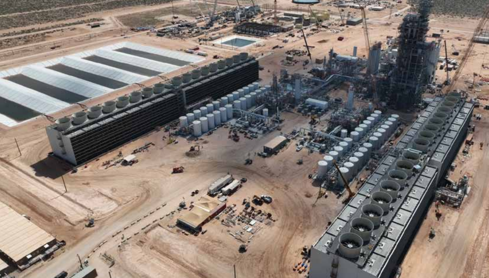
Construction is ongoing for Oxy's massive Stratos direct air capture plant in the Midland Basin, which would represent the first of its kind in the North American oil and gas sector.
