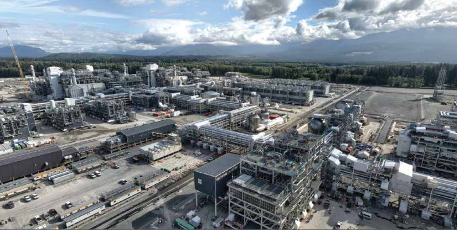
LNG Canada construction activities in August. New LNG projects coming online, including LNG Canada, provide much-needed additional egress options for Canadian LNG export, and increases investment opportunities in the Montney Shale.
