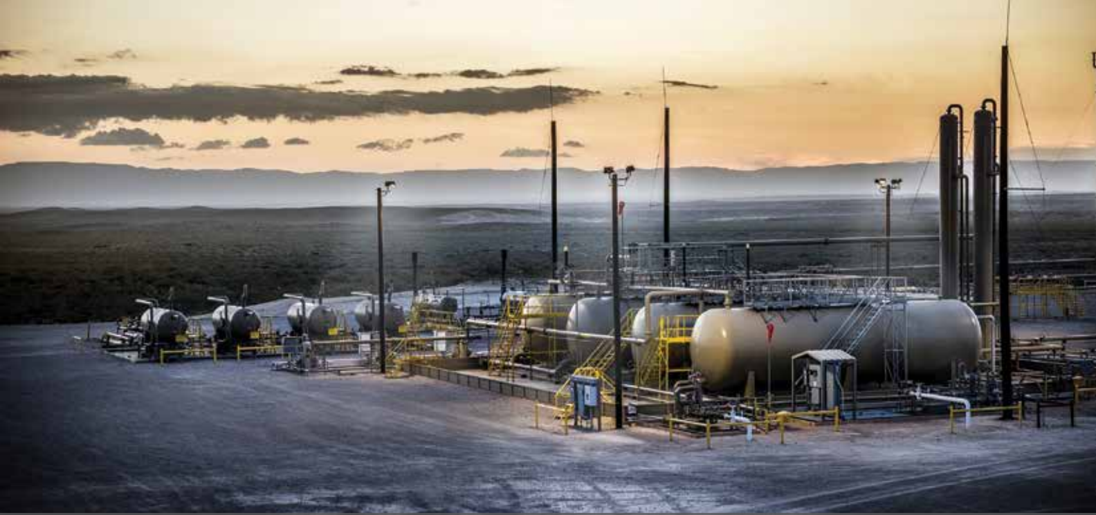
A Coterra Energy pad in the Delaware Basin, including a large tank battery.
